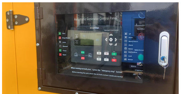
(Customized control module)
